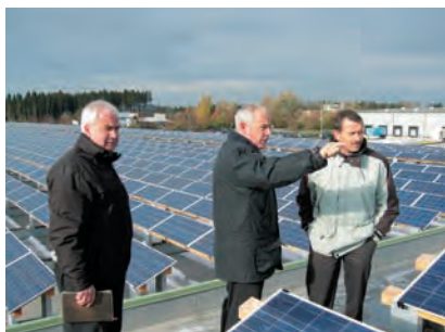
Left: A 450 kW system on the Lebert Company's industrial building; Erbach, Bavaria, Germany.
